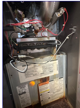
The furnace, cover off
