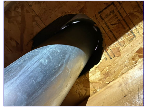
Light coming in from around the HVAC pipe going through the roof. Recommend resealing around the pipe to stop any water intrusion.
