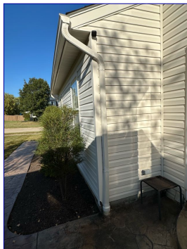
There is vegetation in contact with the house. Recommend trimming trees/vegetation, so it is doesn't come into contact with the home.
