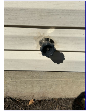
East exterior wall next to gas meter. Hose bib was not tested due to water being shut off in the basement.
