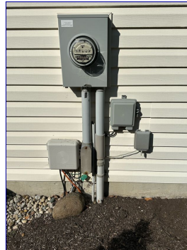
Electrical service entrance located on East side of house.
