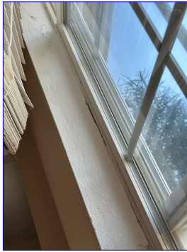
Missing caulk and peeling paint on the interior of the right garage window.
