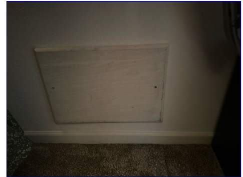
Jacuzzi tub access panel located in master walk-in closet.
