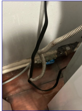
Gas dryer line.
