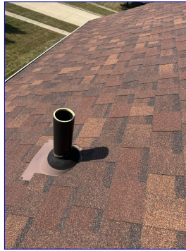
The Plumbing Vent(s)
