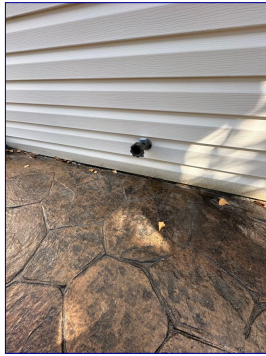
Hose bib on southside of Home, back patio.
