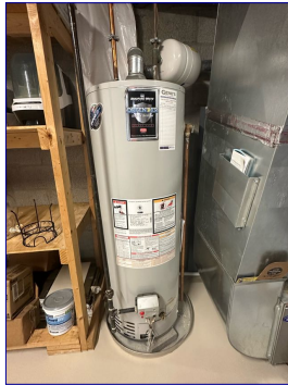
The Water Heater Area
