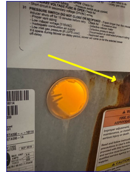
There is rust in the furnace. Recommend a licensed HVAC technician evaluate and repair as needed.
